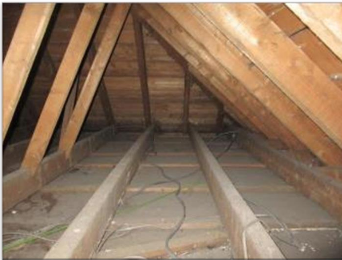
Figure 1 - Uninsulated void in ceiling
